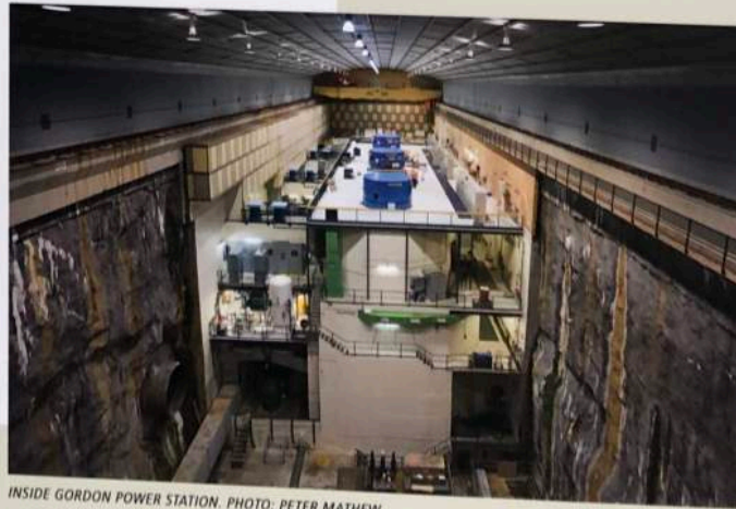
INSIDE GORDON POWER STATION. PHOTO: PETER MATHEW
